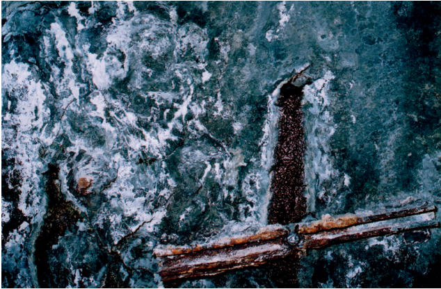
Fig. 7. Salt accumulations (principally thenardite with subordinate gypsum) on the walls of the Cruachan underground power station, Scotland. (Width of field of view c. 1 m). These sulphate salts have formed by evaporation to dryness of groundwater entering the facility, in which the air is heated by operation of hydro-power turbines. (Note the small seepage of groundwater (dark in colour) from a former rock-blot hole, and the badly corroded face plate in the lower right of the field of view; these illustrate the challenge of salt-assisted corrosion in underground voids maintained open for several decades.)
