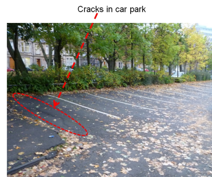
Fig. 2. Photograph showing the crack in the car park.
