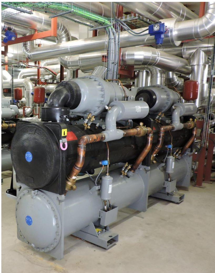
A seriously large heat pump used to extract heating and cooling from mine water at a hospital in Mieres, Spain. Photo by © David Banks
