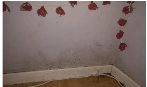
Fig. 4. Mould creeping into Amanda's flat, running from the window down the wall with dark circular marks on the wall leftover prints from Amanda's attempts to '[wipe] it down'.
