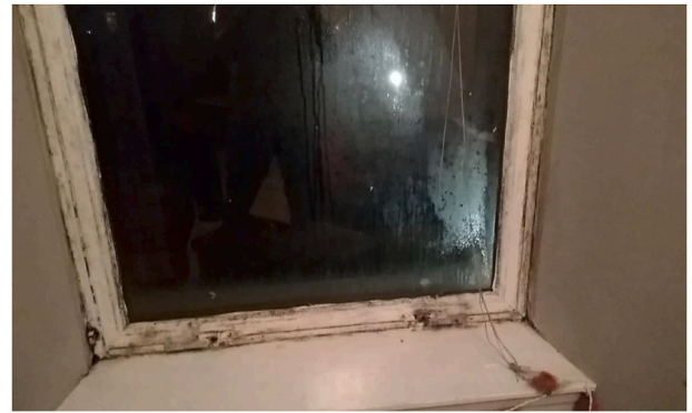
Fig. 3. Mould and condensation forming around Amanda's windowpane.
