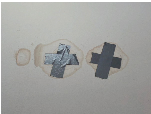
Fig. 1. Watermarks stretching beyond tape placed on the ceiling to try and keep water out (Charlotte, student in her 20’s, living in social housing).
