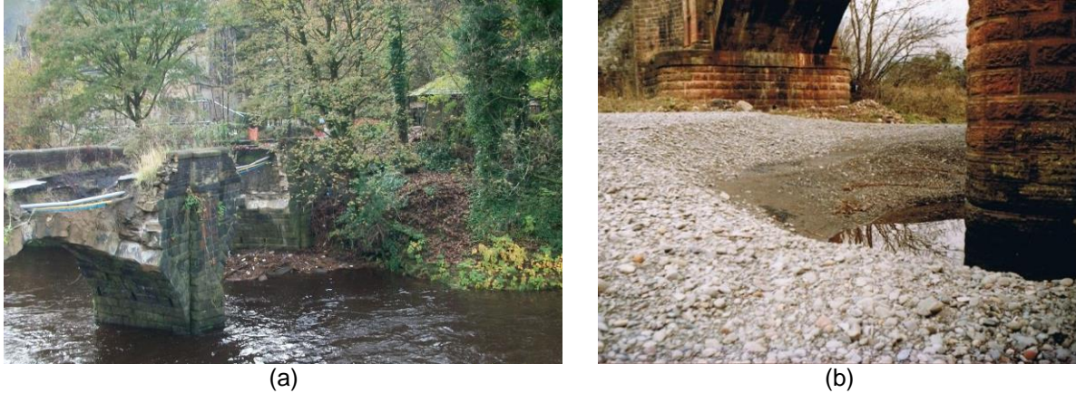
Figure 1. (a) Copley bridge (Halifax, UK) failure due to scour (courtesy of Calderdale Metropolitan Borough Council), and (b) detail of scour hole around a bridge pier [1]
