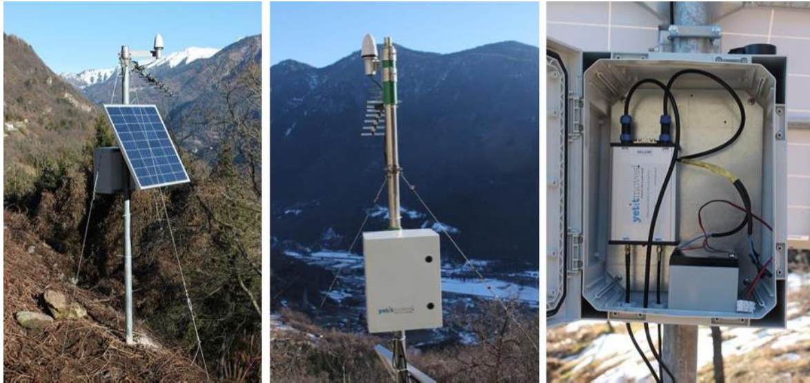
Figure 22. DISPLAYCE stations mounted on the ground in areas subject to landslide. In the photos the receiver and the battery housed in a cabinet with IP67 protection anchored to a pole through suitable fixing brackets [85].
