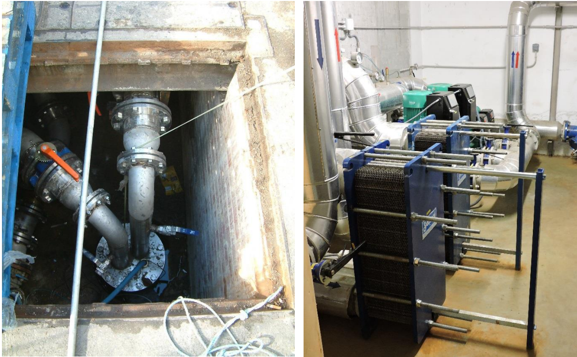
Figure 3. Two components of an open loop ground source heat system: (left) a water well - in this case installed with a submersible pump and reinjection main capable of abstracting/recharging up to 20 L/s (photo © David Birks) and (right) two plate heat exchangers (photo © David Banks).
