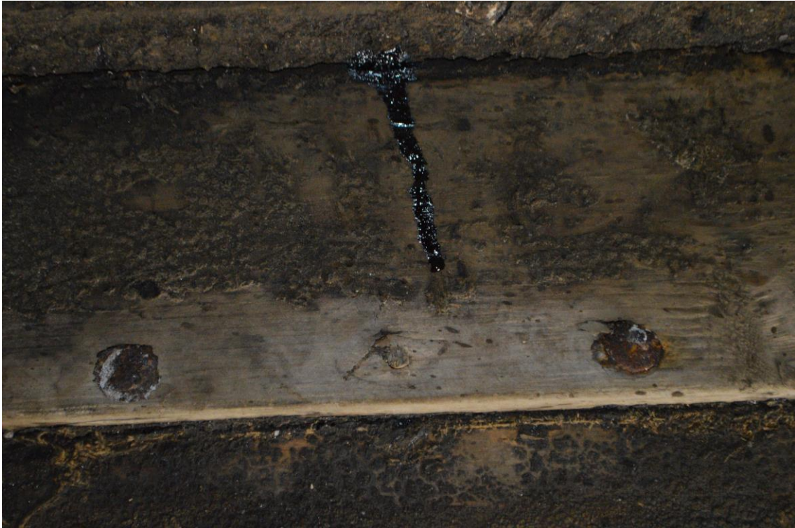
Figure 13 – Replaced planking fastened with round roves. Note the imprints of the original diamond rove fastenings with the nail holes plugged. (Photograph author, Marc Chivers).
