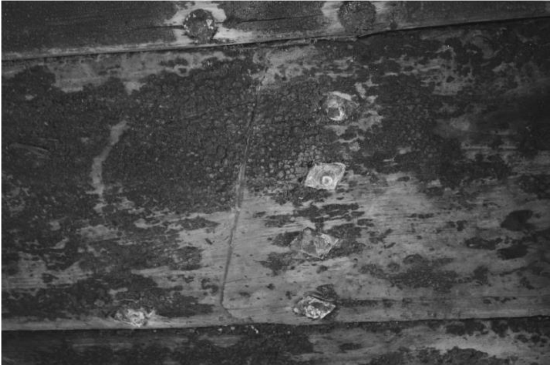
Figure 10 – Evidence of original galvanized fastenings. (Photograph author, Marc Chivers).
