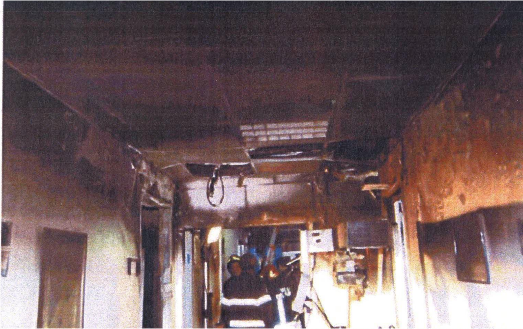
Figure 1: Corridor of the ICU after the fire event (photo by Vatican City Fire Brigade)
