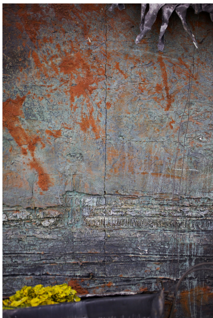
Figure 1 Antonin Artaud Heliogabalus , panel join crack. © Amy Griffin
