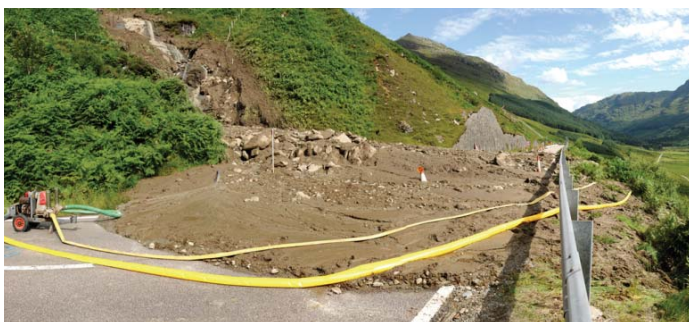
Landslide debris blocking the A83, Rest and Be Thankful, August 2012. Image © NERC
