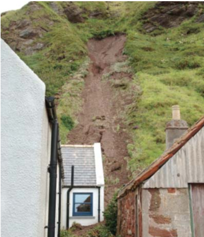
A property is partially buried by a mudslide in Pennan, Aberdeenshire, August 2007. Image ©NERC
