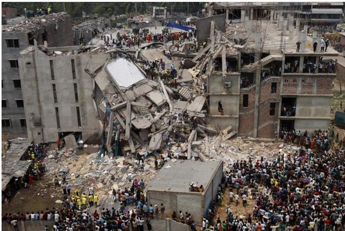
Figure 1: ‘2013 Rana Plaza Building Collapse’, Rijans 007 (2013)
